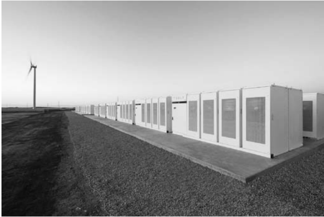
Figure 1. The 100MW Lithium-battery farm set up on 10,000 square meters of land has enough storage capacity to power more than 30,000 homes in South Australia.
